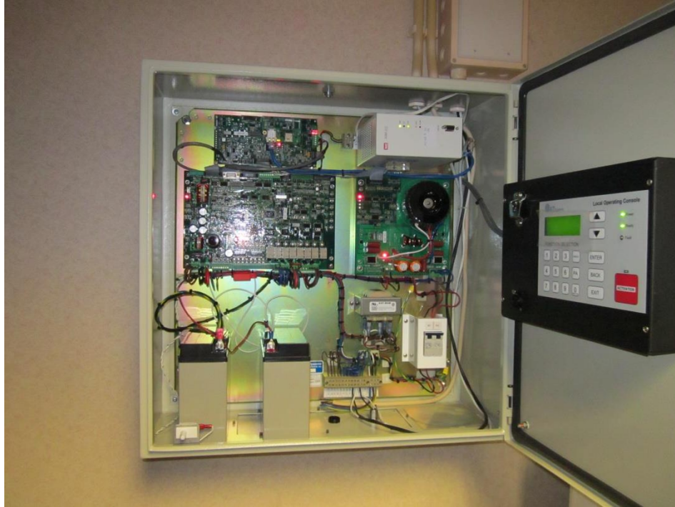
ATI Systems' ISU installed at Lajes Field AFB
