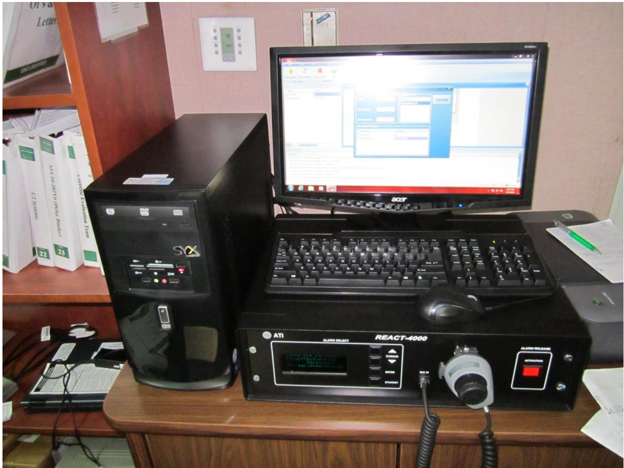
One of the two Control Stations installed at the base
