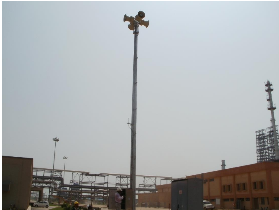
Technician working on an ATI HPSS16 at the refinery
